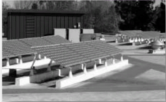
BIA/Sherman Indian School's Hybrid Photovoltaic System Source: DOE
